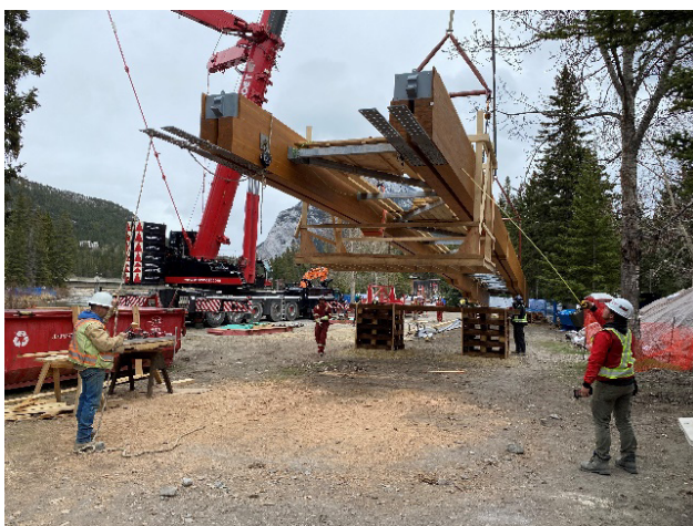
Figure 17 - South section ready for install. Note central pin connection and straps for moment continuity. Credit: Paul Zizka Photography
