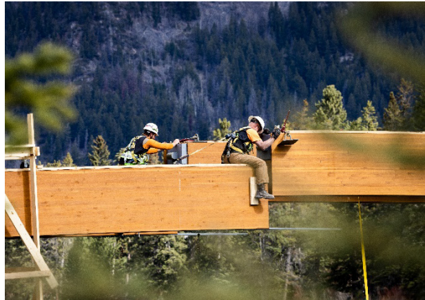
Figure 19 – A central pin locks the two bridge sections together. Credit: Paul Zizka Photography
